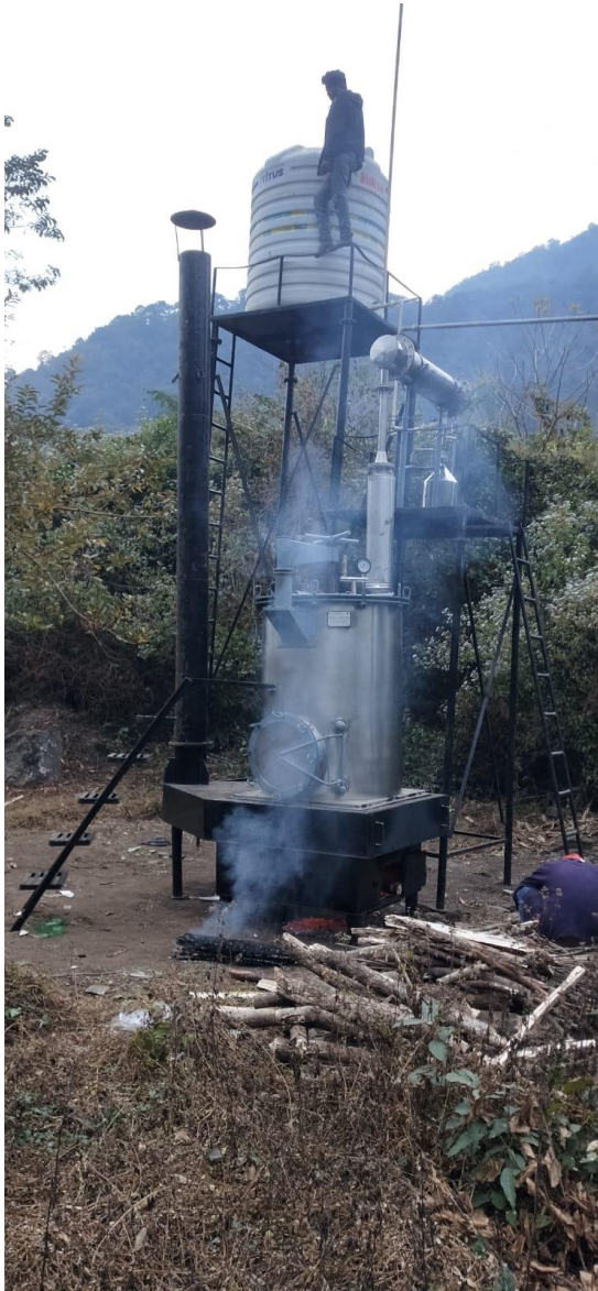
Field distillation unit
