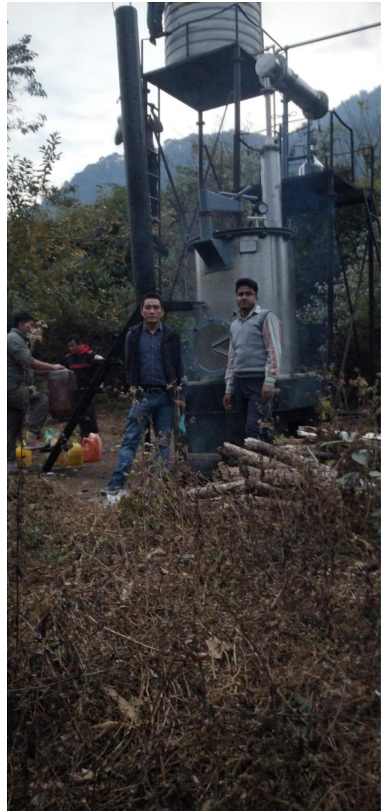
Field distillation unit
