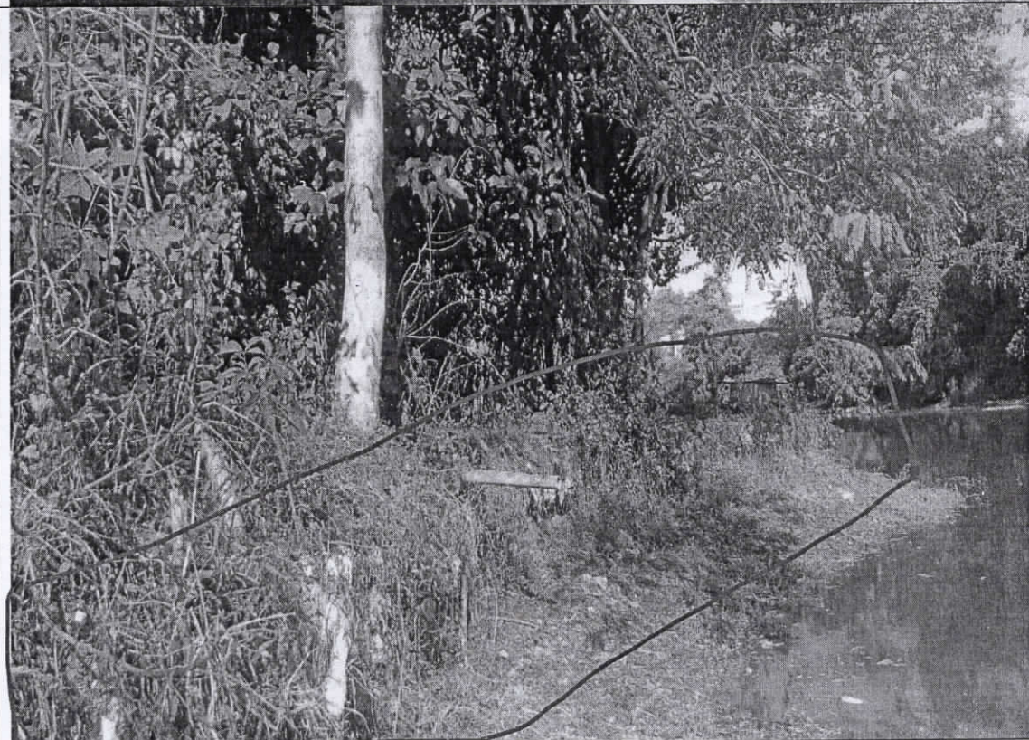
SOIL EROSION IN THE BANK OF THE WATER BODY LOCATED IN FRONT OF VC'S RESIDENCE
